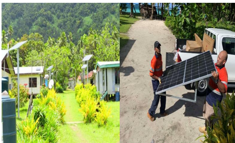
Figure 4.4.3.6 Solar Power Installation
