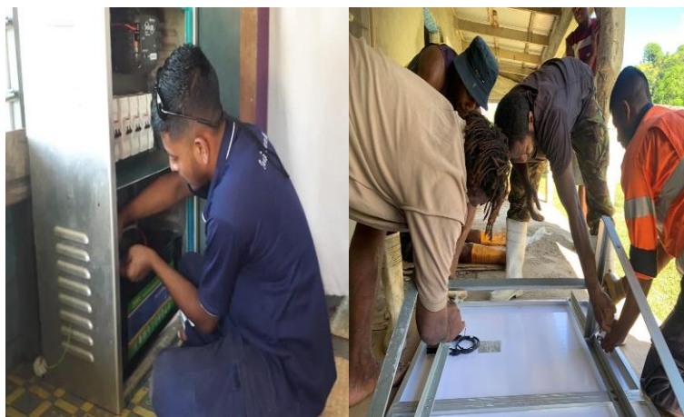
Figure 4.4.3.9 Solar Home Systems Maintenance
