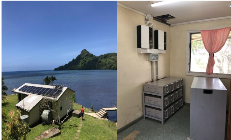
Figure 4.4.3.16 Solarization of Health Centers
