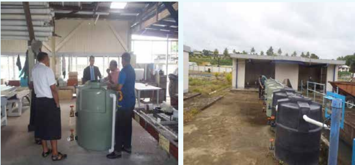
Figure 11: On Left Mr Paul Bayley discussing Advanced Septic Tank Model details and on right the model at KSTP
