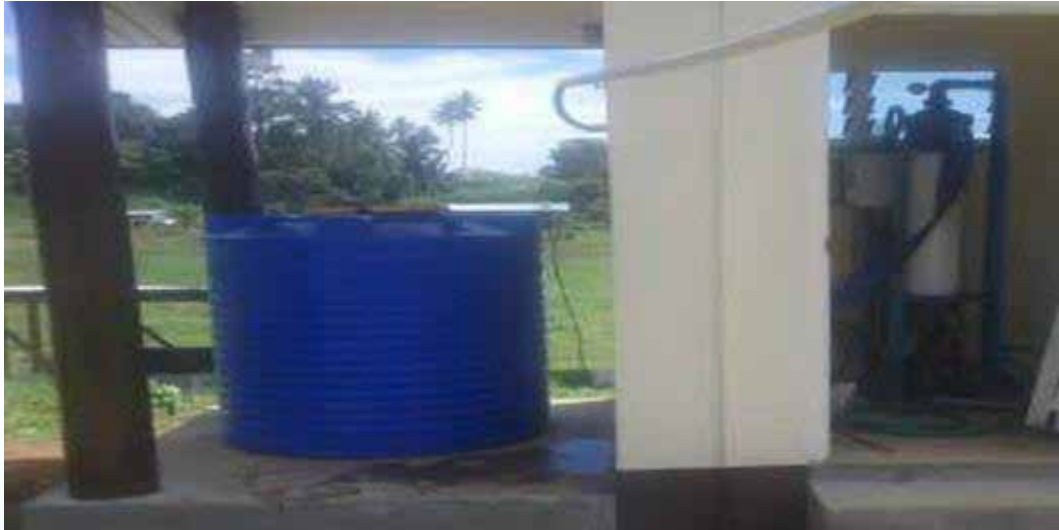
Figure 10: Ultrafiltration Water Treatment System at Tubalevu Village, Tailevu
